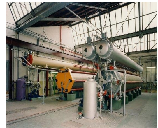
Lurgi High Pressure Elektrolyzer (32 bar)
