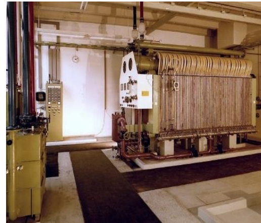
BAMAG Elektrolyzer (atmospheric)
