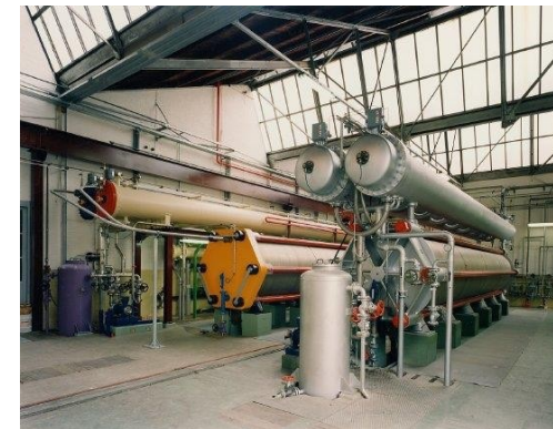
Lurgi Pressure Electrolyse (760 Nm 3 /h; 32 bar)
