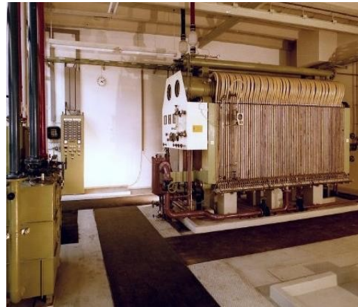
BAMAG Electrolyser (atmospheric)
