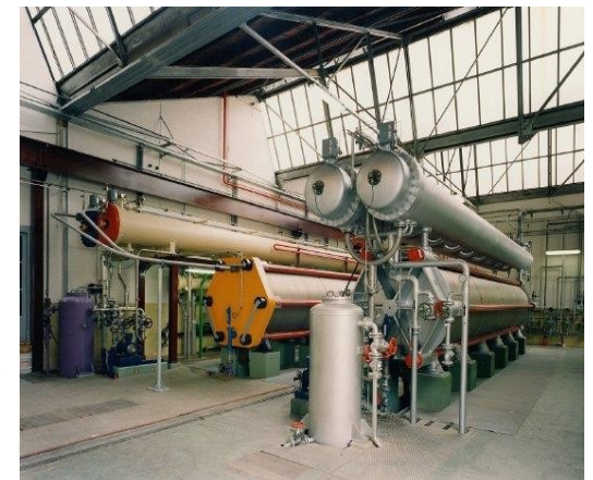
Lurgi High Pressure Electrolyser (32 bar)
